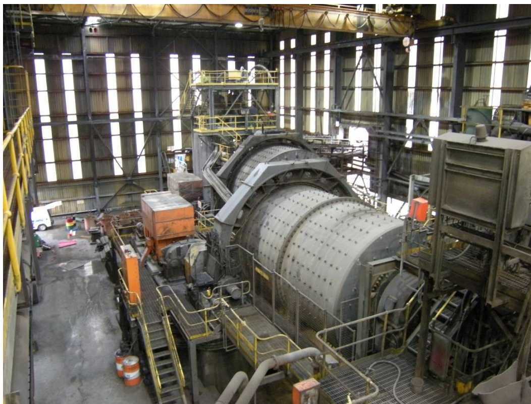
SAG & Ball Mill at the Hellyer Processing Plant
